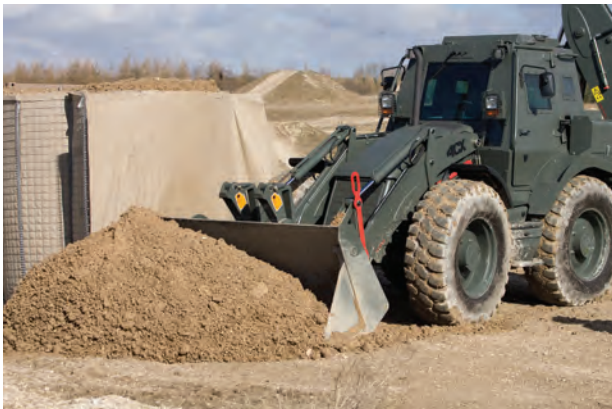
The barriers can be filled with any material in abundance at the site of deployment, reducing logistical concerns.
